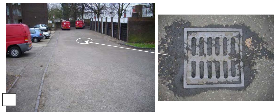
Figure B2 - Example of localised drainage issues: low point at Further Acre and corresponding blocked gully
