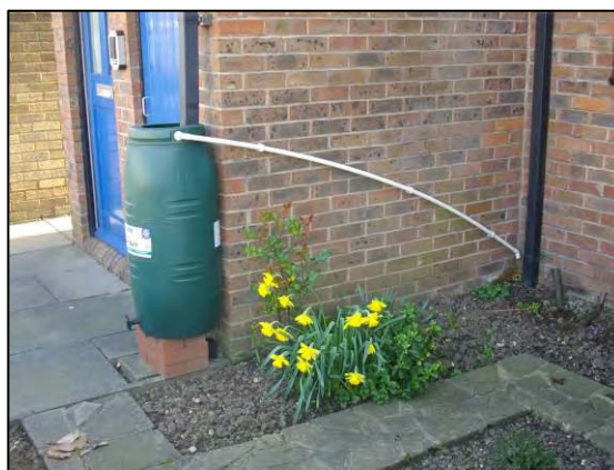
Figure 17 - Example of a 100L water butt in Colindale, in front of the Underground Station
