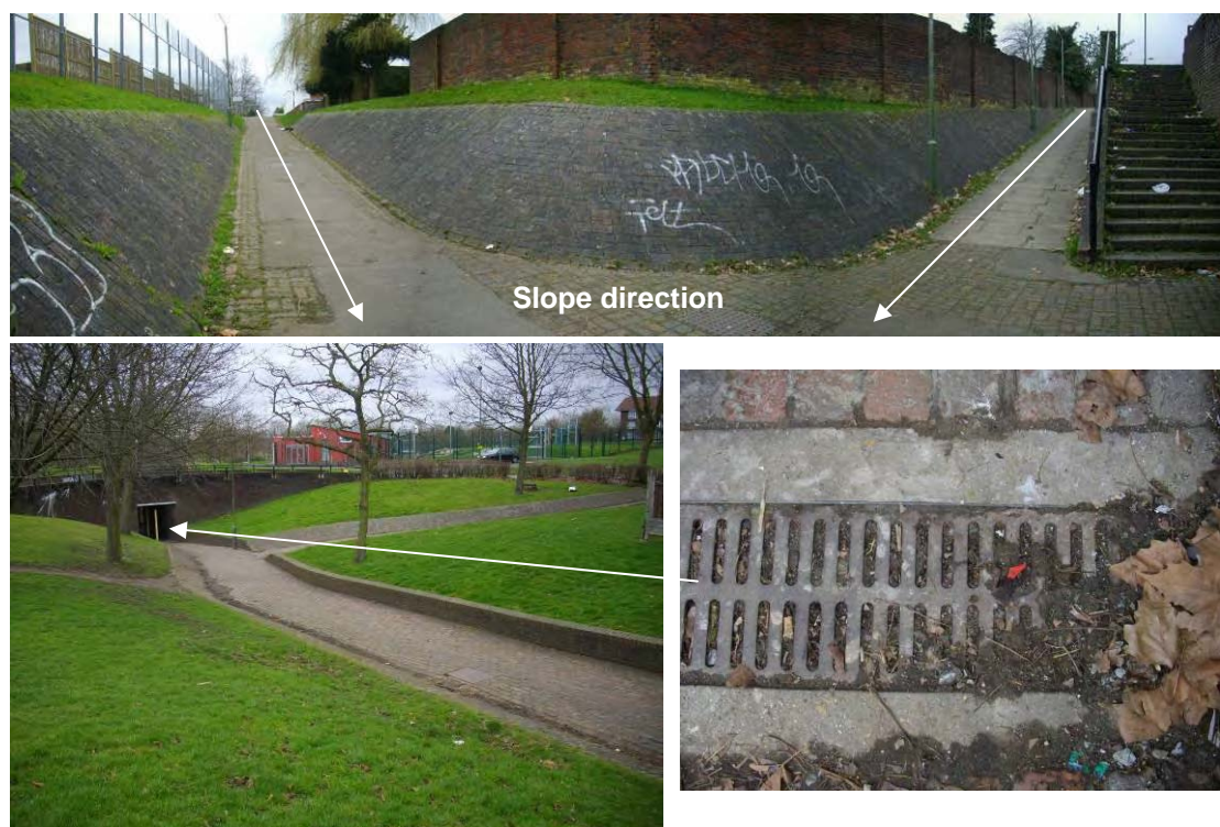
Figure B1 - Example of localised drainage issues: underground footpaths at Grahame Park and corresponding blocked gully
