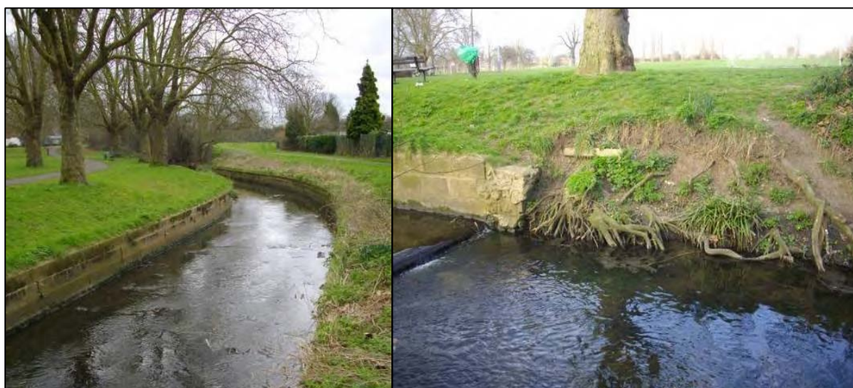
Figure 19 - Pictures of a concrete lined reach of the Silk Stream within the study area, showing erosion (taken 17/03/2009)
