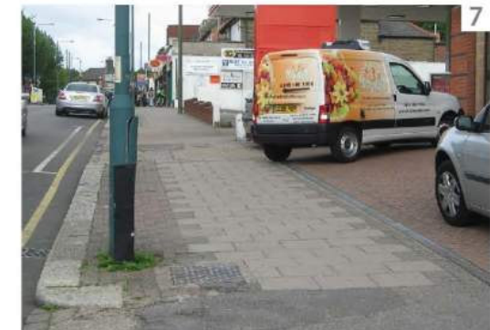
Poor quality, uneven paving
