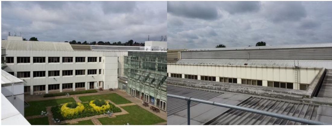
Photographs 8 & 9. Photo 8 (left) shows B1c from B1a. Photo 9 (right) shows the roof of B1c and the joining roof of B1d.
