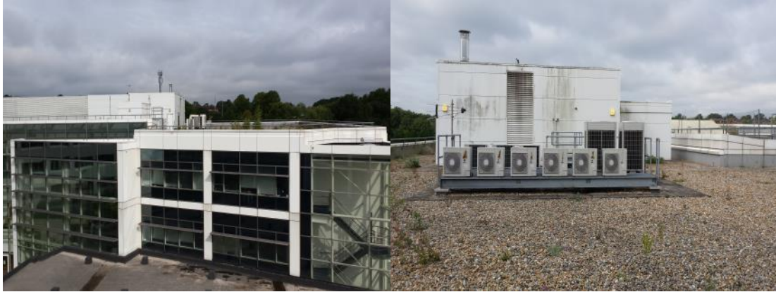
Photographs 6 & 7. Photo 6 (left) shows building B1b from B1a, both have the same construction. Photo 7 (right) shows the roof of B1a, which is similar to B1b.
